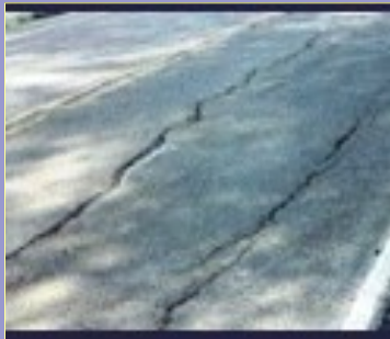
Figure 3: Old worn out road surface: ( Road Science)
