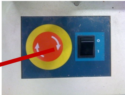
Figure 2. E-Stop and main power switch.
